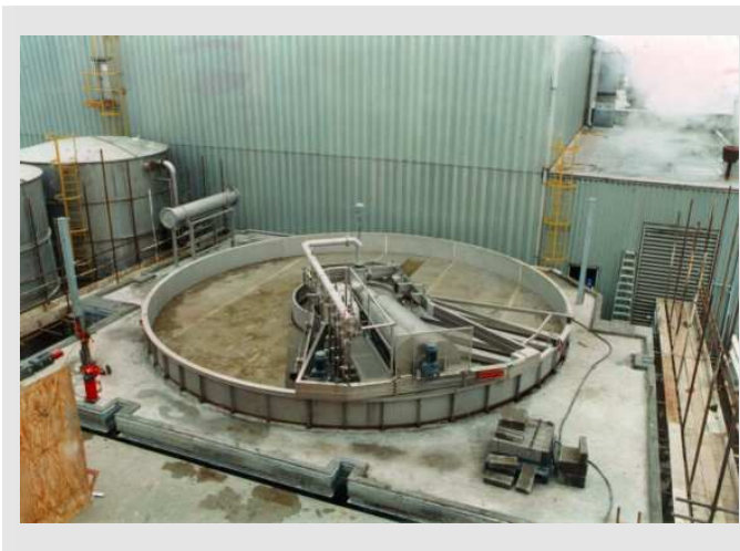
Example for a flotation plant (paper mill)
