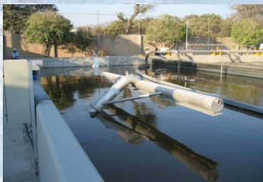
BSK ® -Decanter for discharge of clear water installed at a WWTP in Mexico
