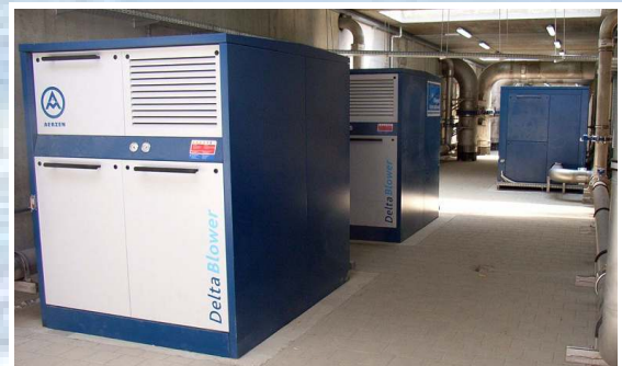
View into the machine room with heavy duty blowers and stainless steel pipe technology.
