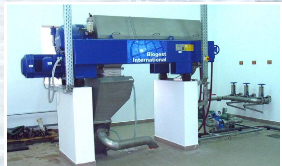
By use of a heavy duty centrifuge excess sludge is dewatered (20 – 30 % DS).
