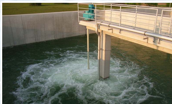
HyperClassic-aeration systems achieve a post-stabilization of the stored excess sludge
