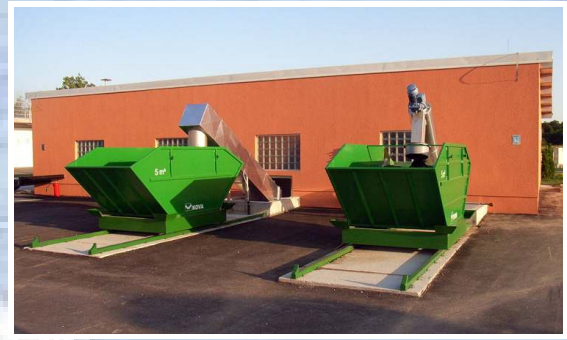
Dropping of sand and solids out of the pre-treatment station. By use of a special washing method, the majority of organic ingredients are led back to the wastewater.
