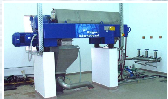
By use of a heavy duty centrifuge excess sludge is dewatered (20 – 30 % DS).
