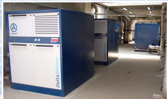
View into the machine room with heavy duty blowers and stainless steel pipe technology.
