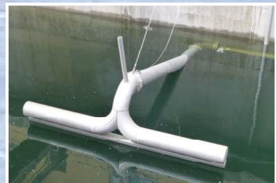
The discharge of clear water is performed by BSK®-decanters
