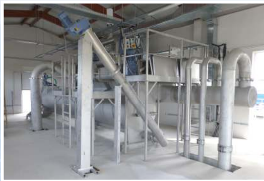
The wastewater enters primary cleaned by pressure pipes the compact pre-treatment station and is in the further process released from fine ingredients, sand and grease.
