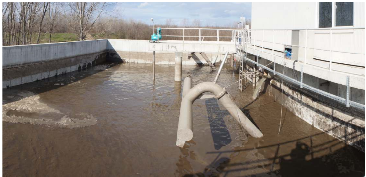
SB-reactor 1 of wastewater treatment plant Kozlodui during fill-up-phase
