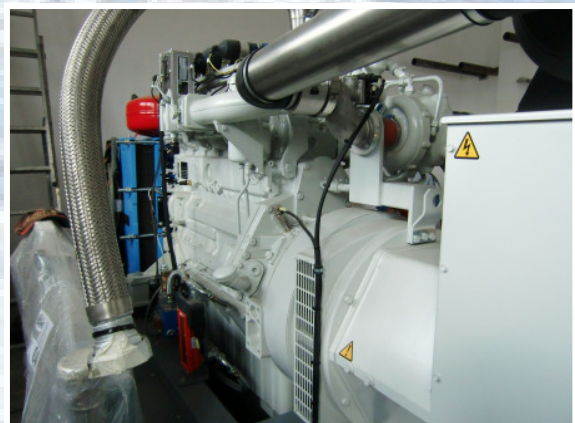
Combined heat and power plant for power generation out of biogas
