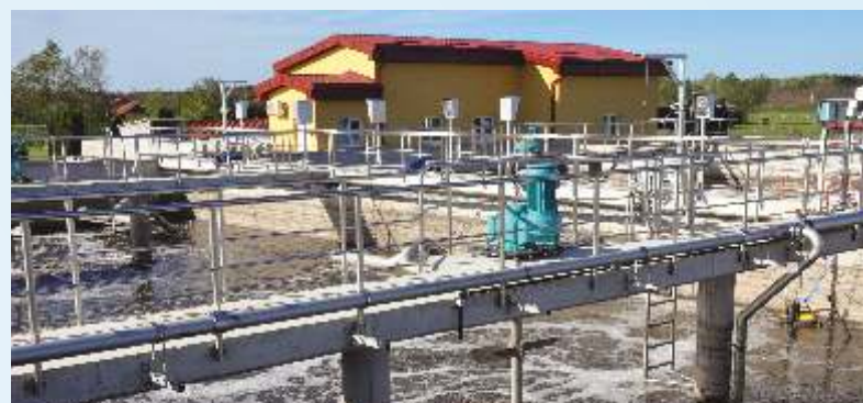
SBR-WWTP of the city of Durdevac (Croatia)
