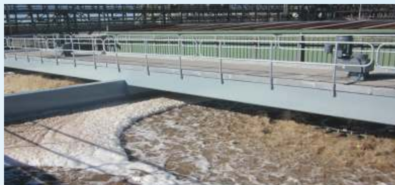
BSK®-Turbines of a paper factory in Spain
