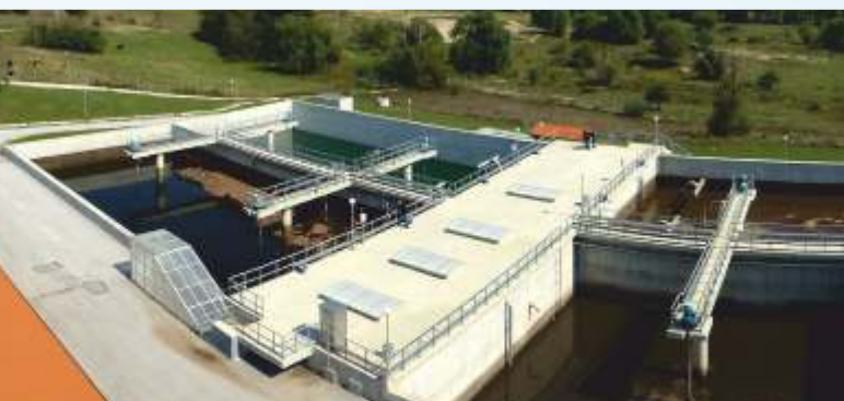
SBR-WWTP of the city of Hisarya (Bulgaria)
