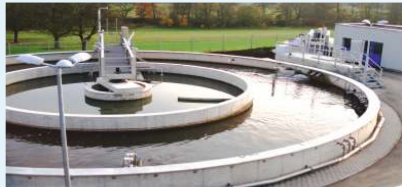
WWTP of Gersheim (Germany)
