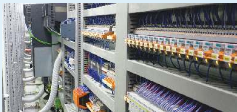
Inner view of the control panel of a WWTP
