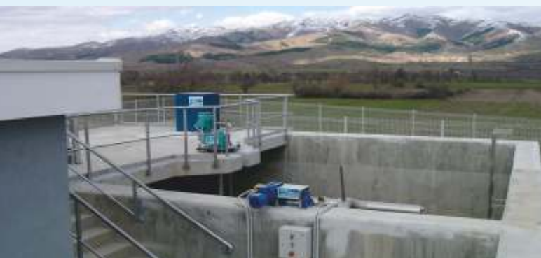
SBR-WWTP of a tobacco factory in Bitola (Macedonia)
