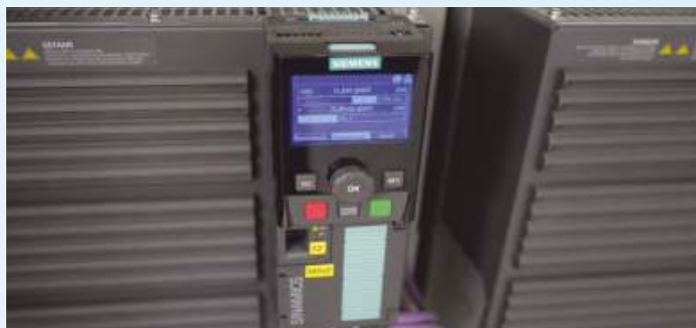
Frequency converter of an electrical drive system
