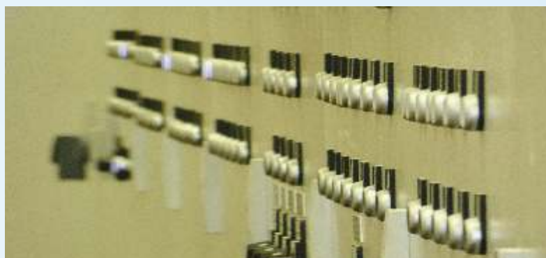
View of the control panel
